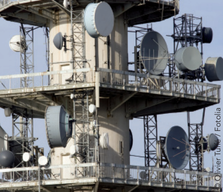
Telecom - Data infrastructure
